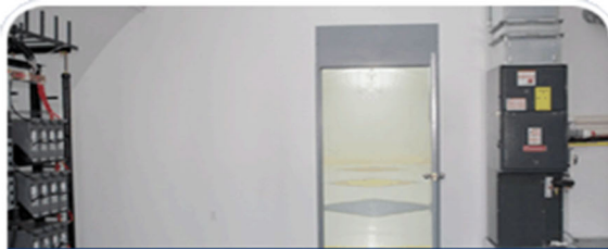
BUNKER MECHANICAL ROOM
