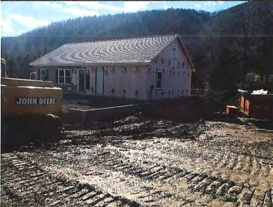
Site visit to 111 Patchen Court 2/27/18 showing partially built home and extent of disturbed soil.
