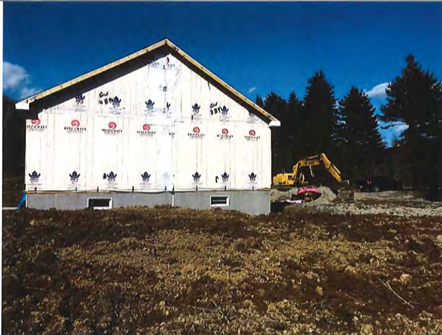
Site visit to 111 Patchen Court 2/27/18 showing disturbed soil throughout the site. Photo taken from deep hole location.
